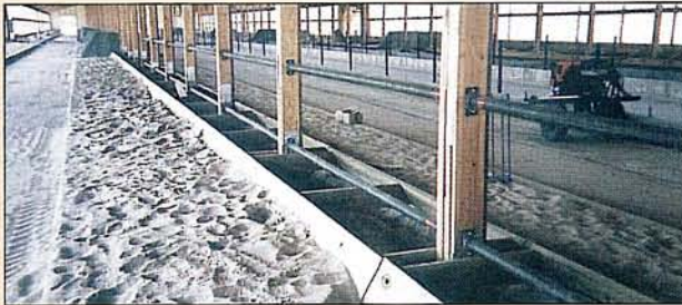
INFRASTRUCTURE being installed in a wood frame barn. NOTE no stub posts needed. Mounts directly to building columns. Horizontal railings will allow for ease of freestall width adjustment to 44", 46", 48" or as desired.
